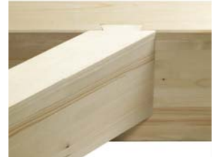
Joist skewed in relation to stringer
